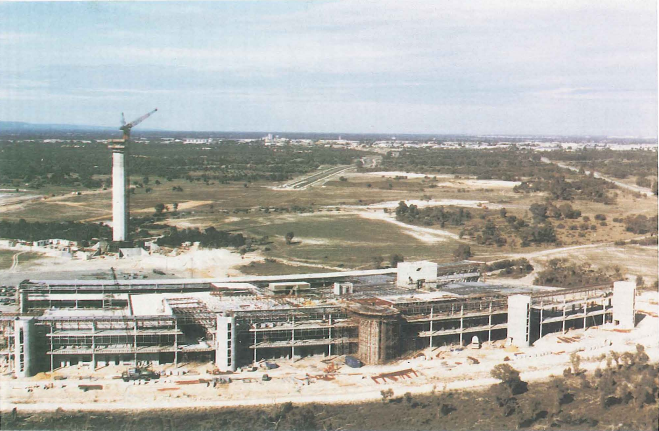
PLATE 13 — The new International Passenger Terminal Building and Control Tower under construction at Perth Airport. The buildings are expected to be operational by September 1986.
